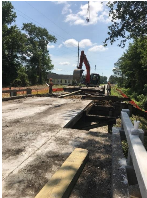
Figure 4.1.3 Concrete Slab from Bridge #10 in Beaufort County, NC, Division 2
