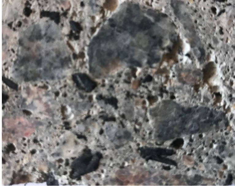
Figure 6.3.4 Missing STR Fine Aggregate Particles on Concrete Surface
