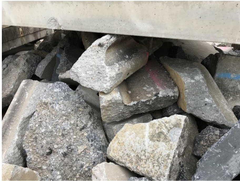
Figure 12.12.14 Concrete Panels Were Broken and Reba Was Removed
