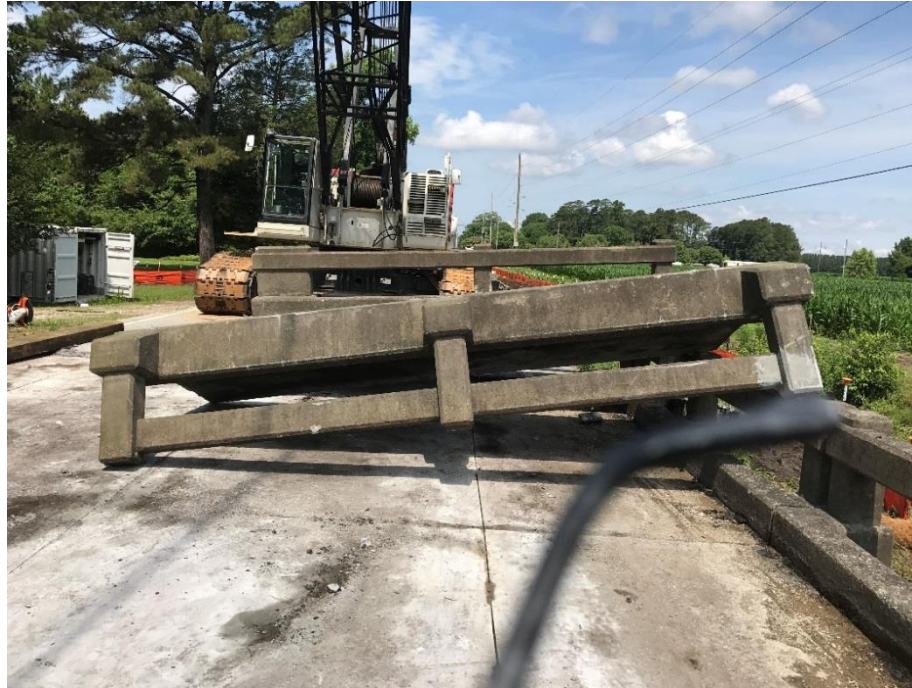
Figure 12.12.3 Concrete Panel Removed – Division 2
