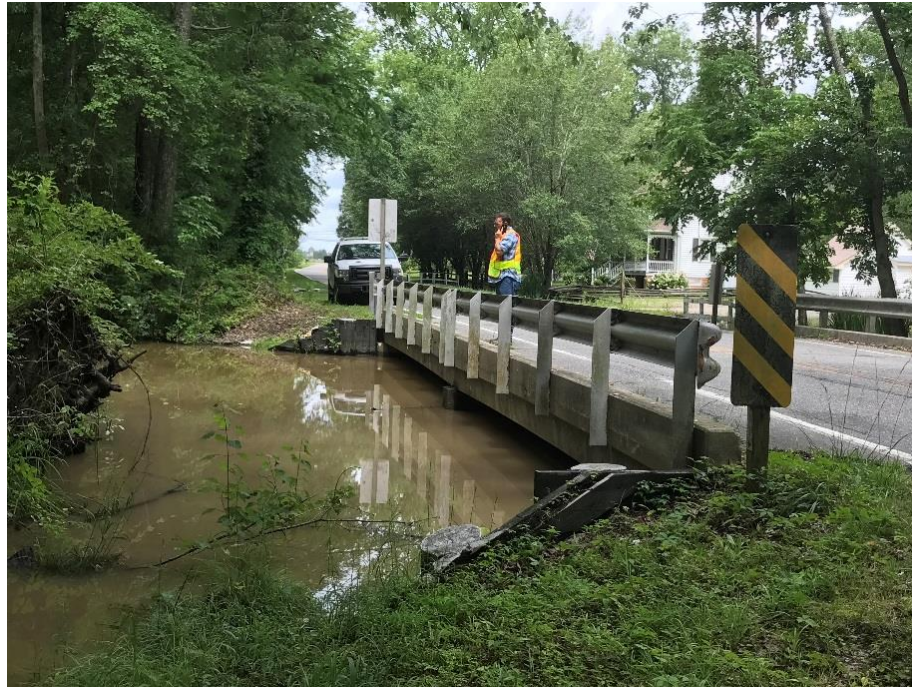
Figure 12.12.1 Bridge Construction Site in Division 1 to identify the Slabs to be Saw Cut
